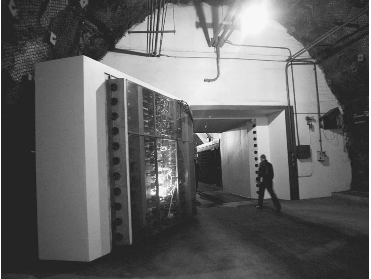
The “steel city” defense complex of the North American Air/Aerospace Defense Command, NORAD, shown in 1997, was carved out of Cheyenne Mountain in Colorado in the early 1960s. Fifteen steel buildings inside the mountain stand on rows of huge steel springs, designed to negate the earthquake effect of a nuclear blast. AP/WIDE WORLD PHOTOS.
